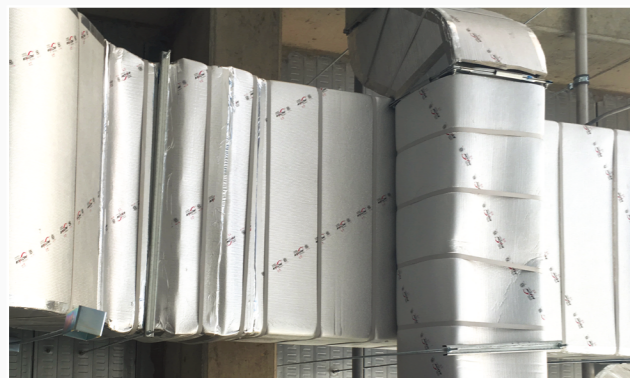
Aluminum foil insulation for DUCT
